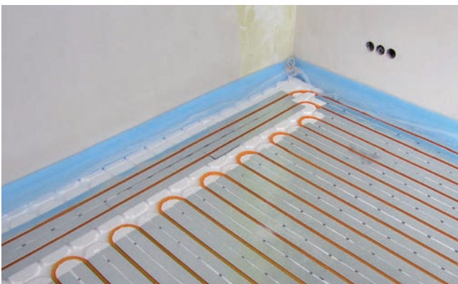
Completed heating system 25
