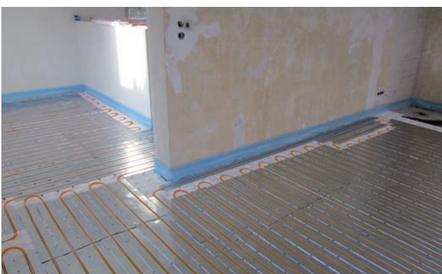
Completed heating system 25
