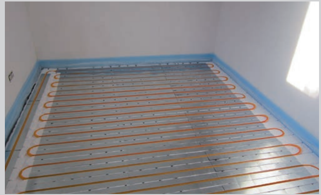
Completed heating system 25
